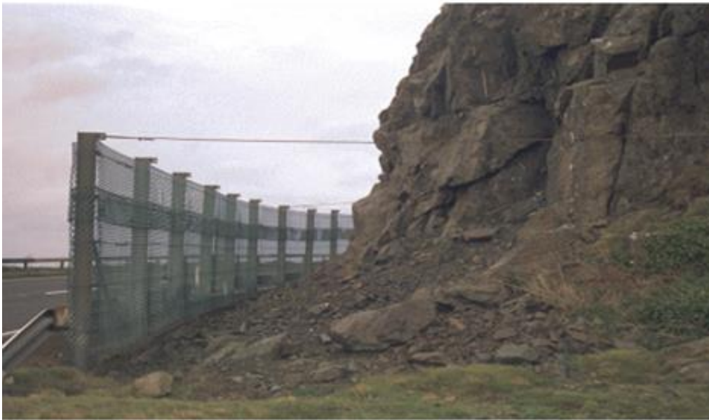
Figure 6.10 Effective Rock Trap Barrier (A77, Ballantrae)
